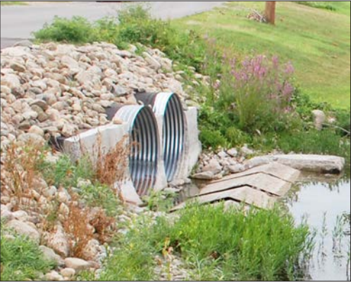
The “lake” side of the Maxinkuckee outlet on the west shore, where drought conditions have left the culverts carrying water to Hawk Lake bone dry.
